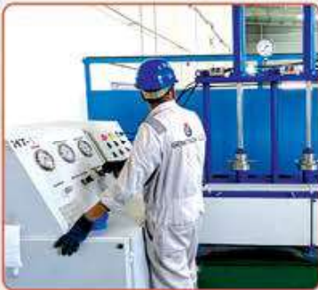
Hydro Test Bench
